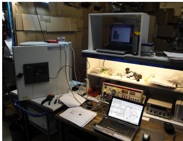
Image 1: Testing the under-voltage dependent directional reactive power relays
